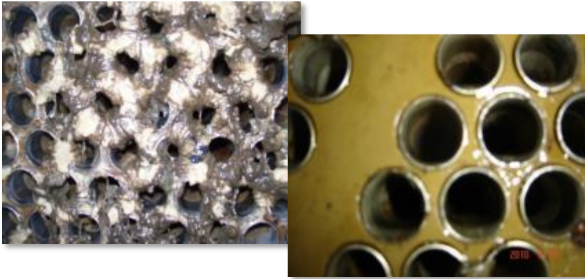
Cooling Tower Condenser Tube Sheet
