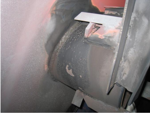
Fig. 5. Two-phase FAC in a deaerator. Photo courtesy of Tom Gilchrist (ret.), Tri-State G&T.
