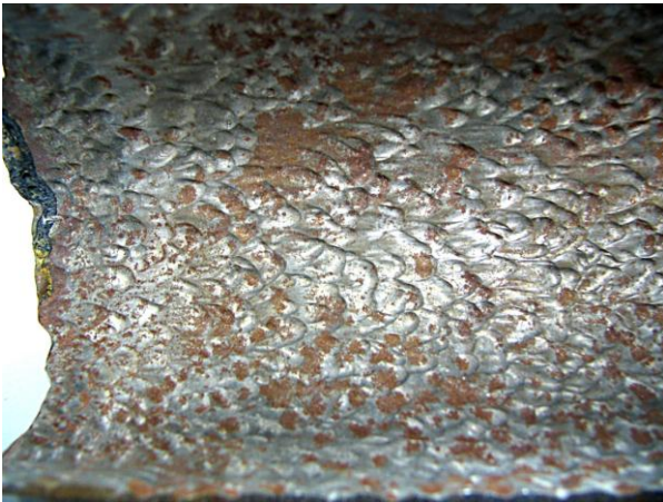
Fig. 1. Single-phase FAC. Note the orange peel texture. Photo courtesy of Dave Johnson, ChemTreat.
