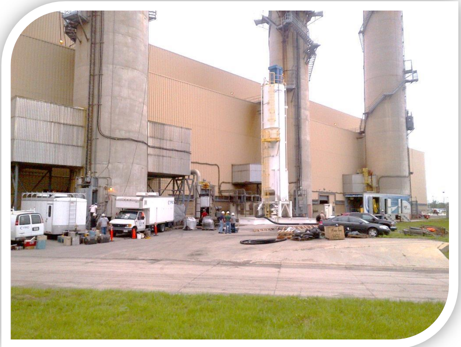
Portable injection systems used for dry sorbent and mercury sorbent injection
