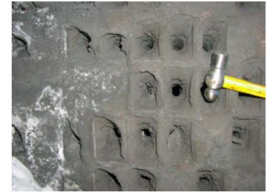
Tube Sheet Fouling
