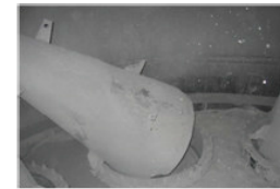
Construction quality finding
