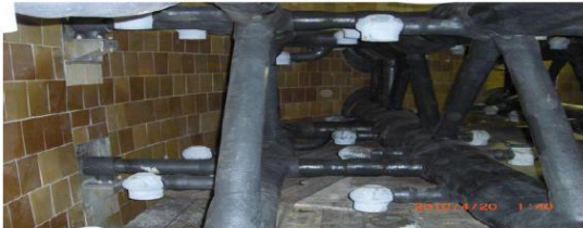
Fig. 7 Typical Spray Headers
