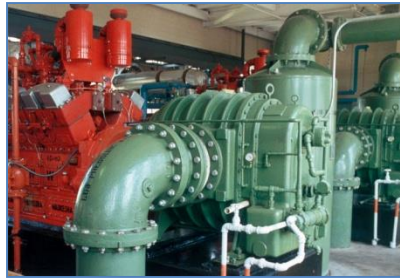
PD Roots Lobe Blower: Lowest efficiency (45-65%), lowest capital cost
