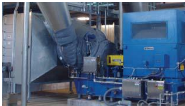
One of three Siemens Turblex KA44-GT315 flue gas desulfurization oxidation air compressors, each 18,000 scfm, 30 psig, 2500hp.
